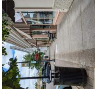
Widening the sidewalk to match the design on the south of Mill St.
